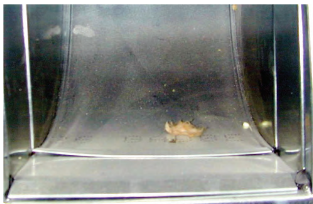
All the white dust consists of SPF dust. This photo was taken in a newly constructed home.
