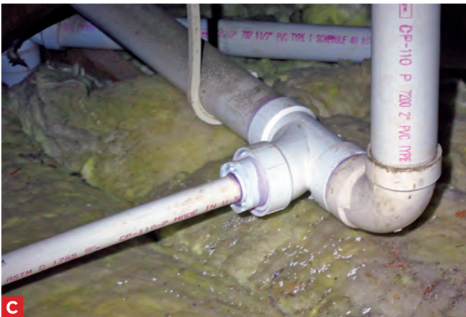
C This attic HVAC condensate line is directly tapped into the sewer vent in the attic. This is not allowed. Sewer gasses will enter the HVAC through the condensate line, which has no trap or air gap.
