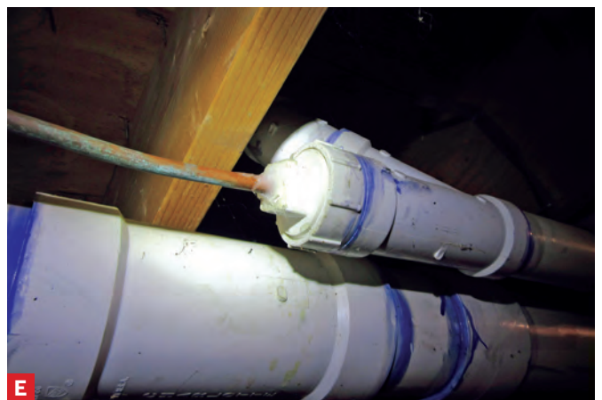
E Another condensate line directly entering the sewer line without a trap or air gap. This one is prone to raw sewage discharge into the condensate line.
