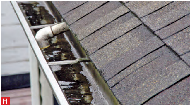
H This is one of the worst condensate disposal methods for attic HVAC units. The contractor drills a hole through the fascia into the gutter. The standing water in the gutter will freeze and prevent discharge of condensate from a heating unit. This can result in a shutdown of the heating unit.
