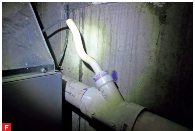
F This HVAC trap is doing nothing. The pre-molded plastic trap is installed so steep there is no trap. There is also no air gap.
