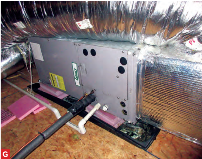
G This condensate drain on the attic HVAC is an example of a trap that cannot be cleaned without cutting the drain. This is prohibited.
