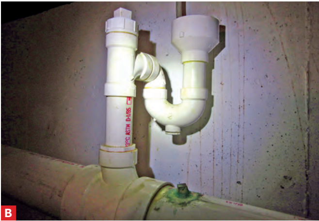
B This is a proper waste receptacle installed on a main domestic sewer line. The drain has a proper trap with a large opening to allow an air gap. Notice the plug just below where the condensate line was previously installed directly into the sewer line. I had inspected this home and called out the improper means of condensate disposal. The homeowner had the system repaired, and I went back to confirm the proper repair.
